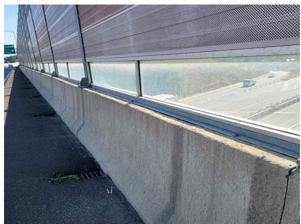
S2 균열 (0.2mm/1.5m×14EA)
