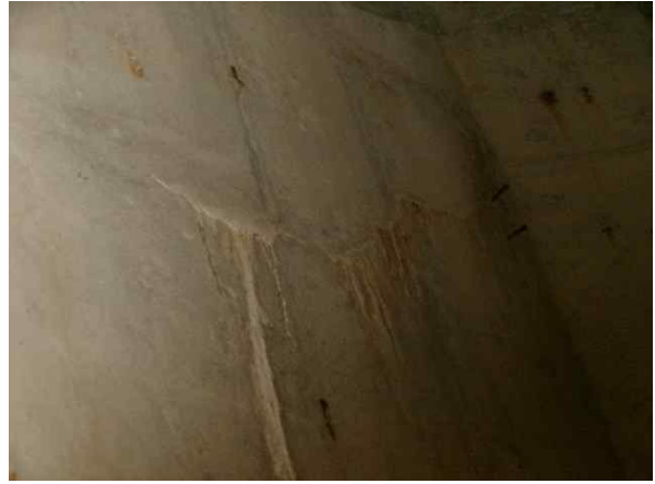
A1 균열부백태 (0.2m x 1.5m)
