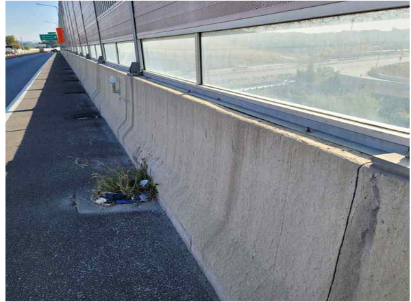
S3 균열 (0.2mm/1.5m×16EA)
