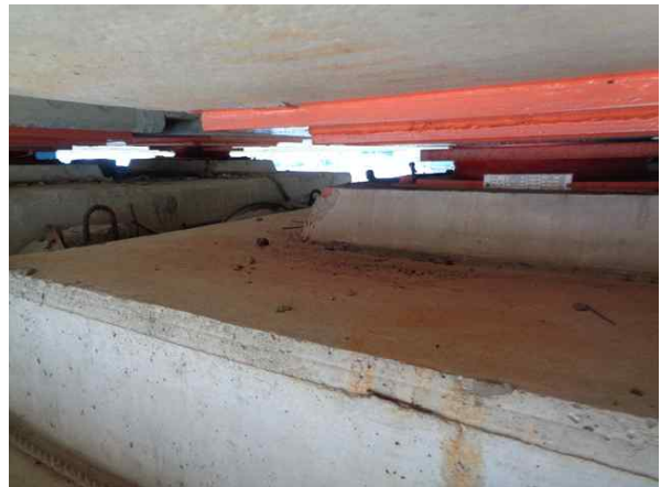
P5-Sh12 받침물탈 파손 (0.1m×0.1m)
