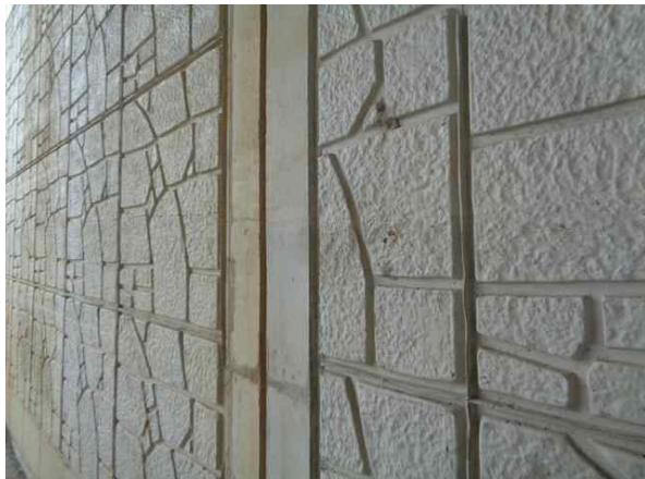
A2 균열 (0.2mm/3.0m)
