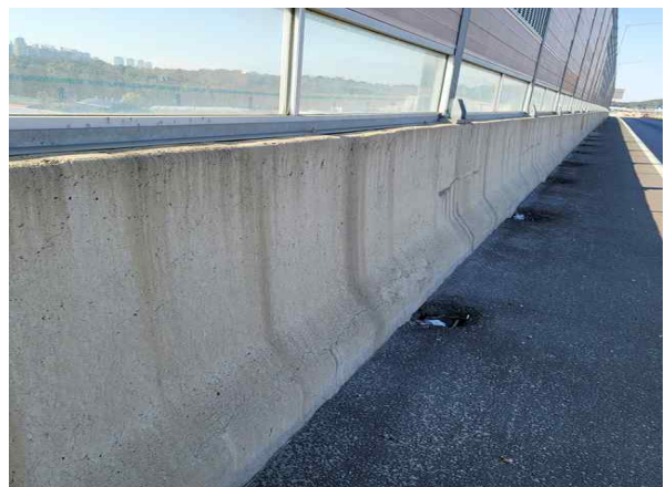
S5 균열 (0.2mm/1.5m×24EA)
