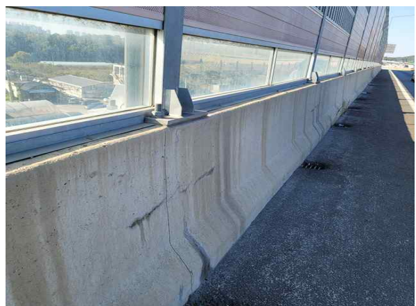
S6 균열 (0.2mm/1.5m×12EA)
